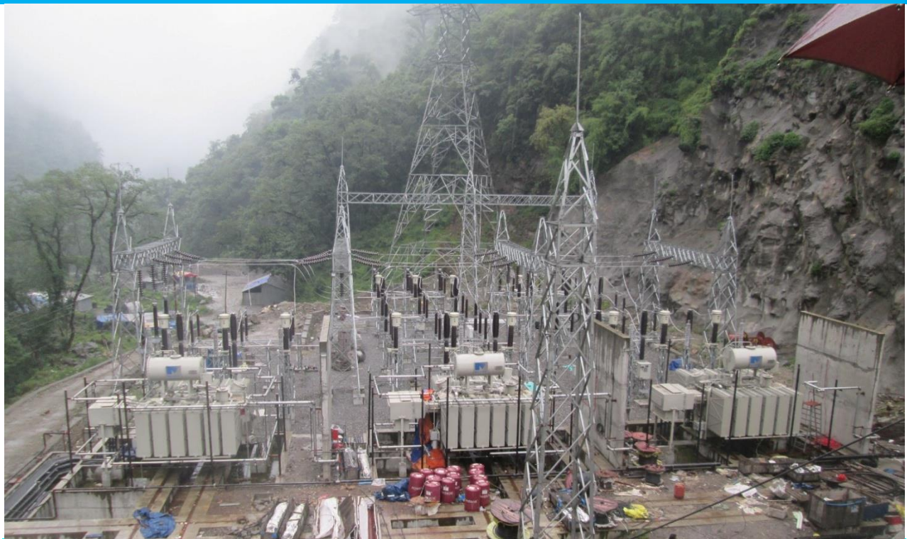
Sending End Switchyard
