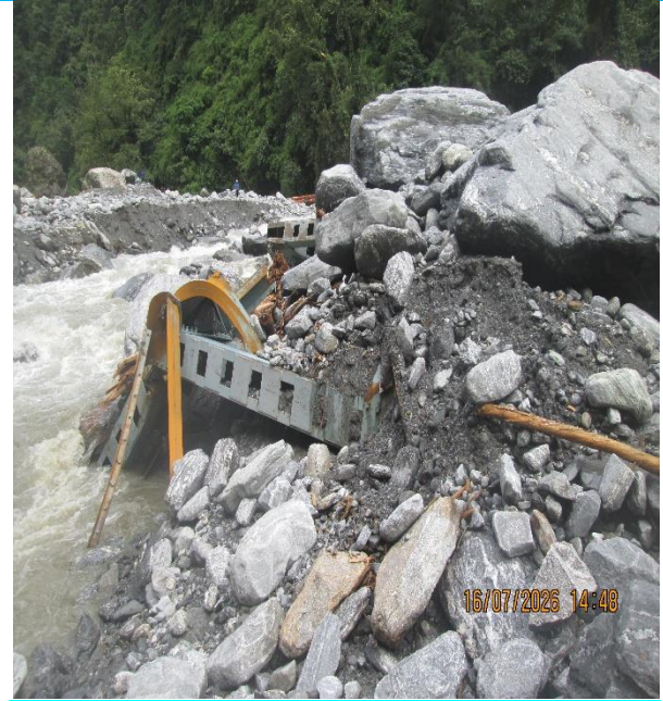
Impact of Flood overturning Main Access Bridge
