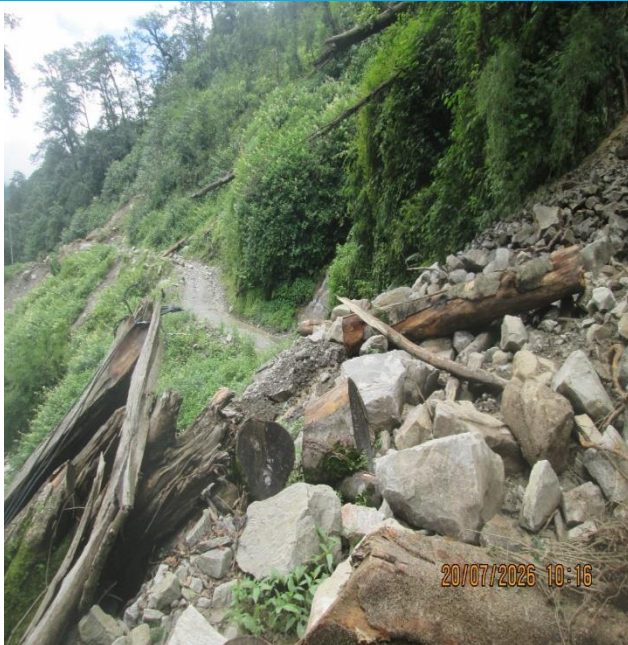
Impact of Landslide in Access road
