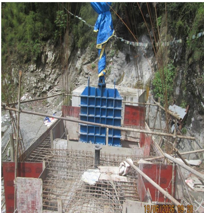
Knife Gate Valve at the Likhu Inlet Tunnel
