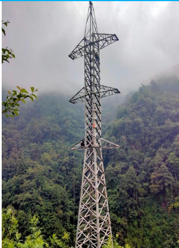
AP1 Transmission Tower
