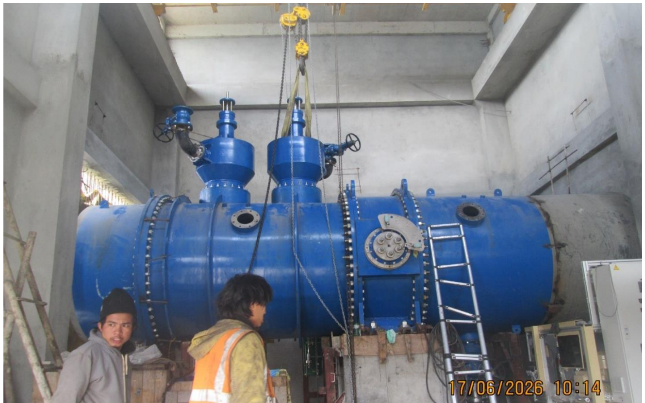
Pressure Protection Valve (PPV) at Outlet
