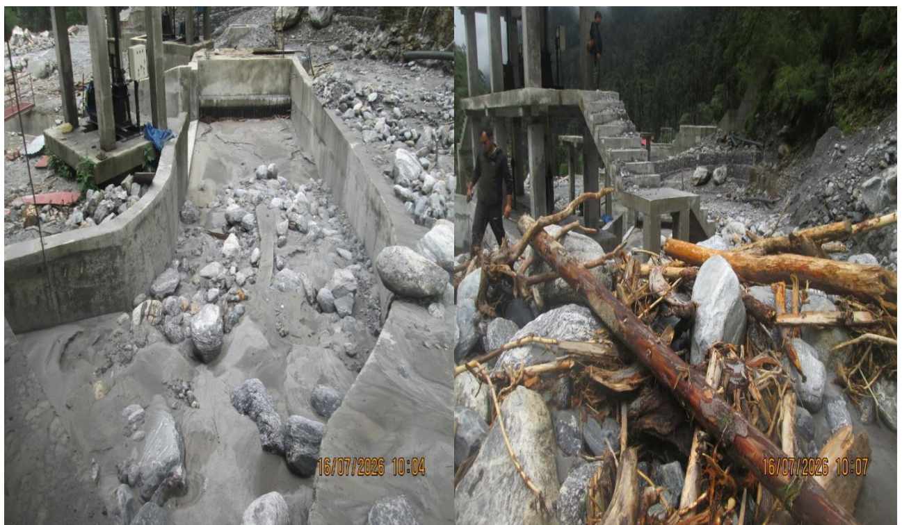
Impact of Landslide at Likhu headworks
