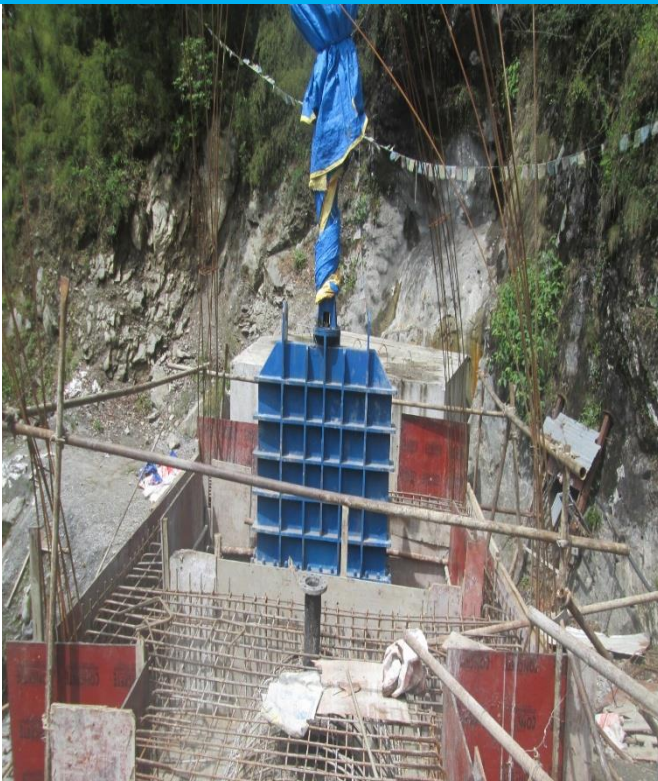
Knife Gate Valve at the Likhu Inlet Tunnel
