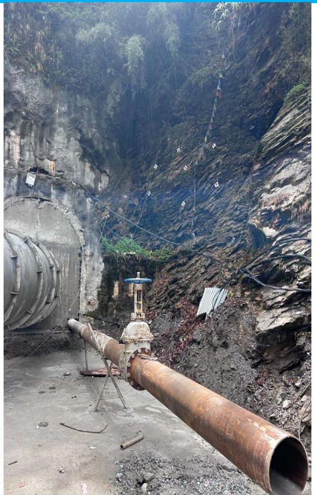
Valve works at Nupche Portal
