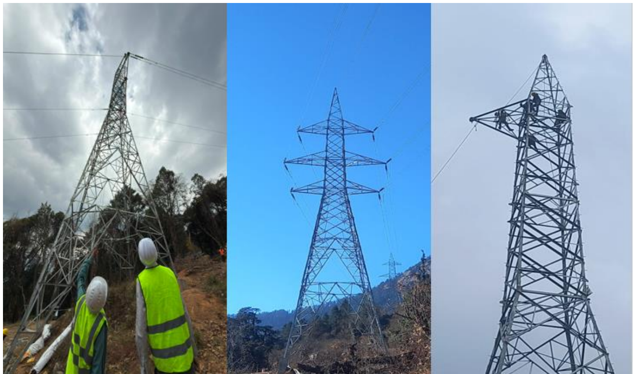
NLHP Transmission Line Towers
