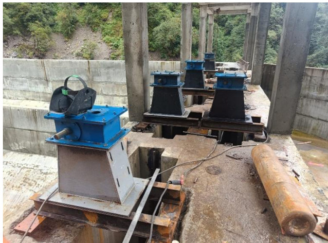
Gate Hoisting System Base
