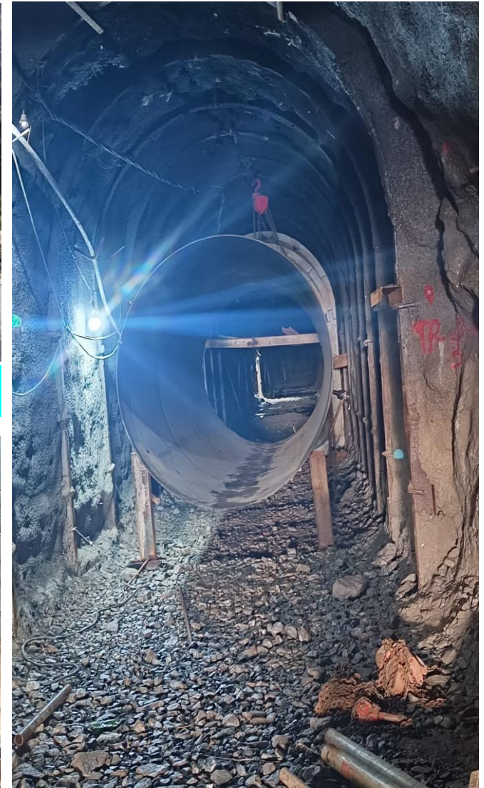
Penstock Pipe Alignment
