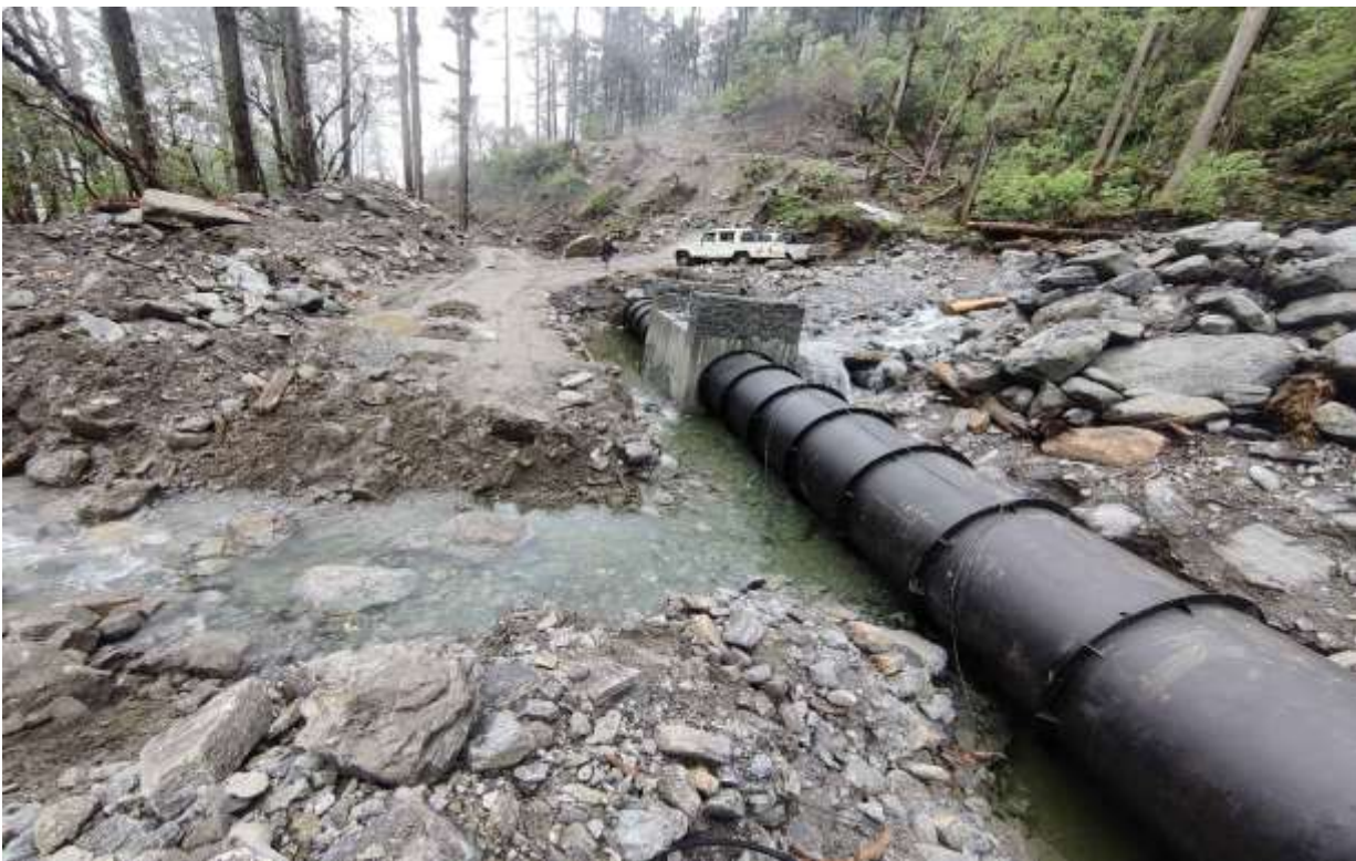
Likhu Headrace Pipe
