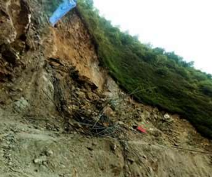
Landslide in Surge Shaft area
